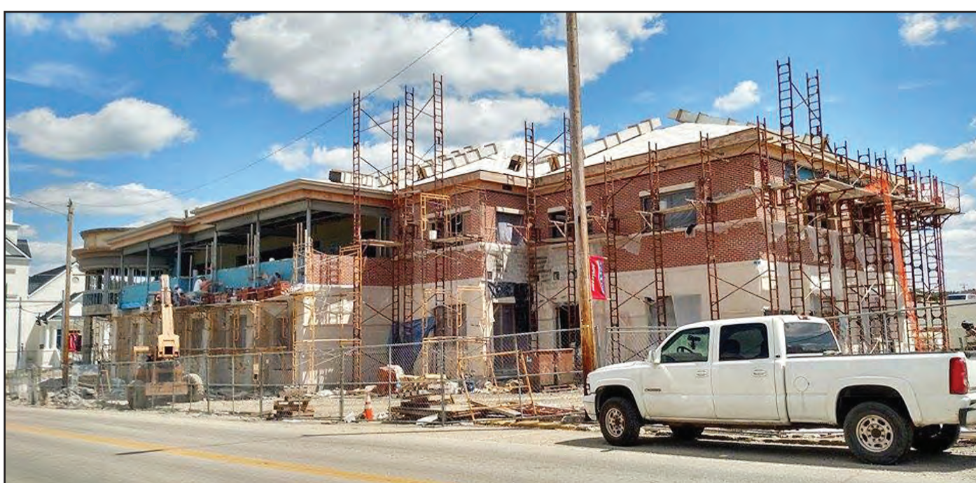
Pictured above is the Commercial Bank construction site on Main Street. Bank officials say the building is approximately 66 percent finished and estimate that construction could be complete in December. (Photo by Jim Gazay)
