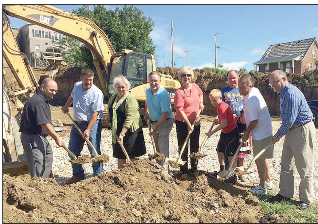
City officials broke ground last Friday on a new parking area located between Trimble Street and Riverside Drive. Mayor Mark Walter said at last week's Chamber of Commerce meeting that the two-tier parking will include 12-14 spaces off Trimble Street and 54 spaces off Riverside Drive. Pictured above left to right are city council members Tristan Daniel and Carter Bolin, Gail Wright of Gateway Area Development District, Mayor Mark Walter, city council member Phyllis Keeton, John Standafer (contractor) and son Riley, city council member Dwayne Nickell and Mark Collier of Gateway Area Development District.
